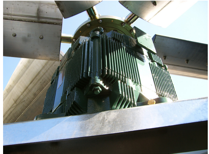
Direct drive motor in a Marley NC cooling tower
